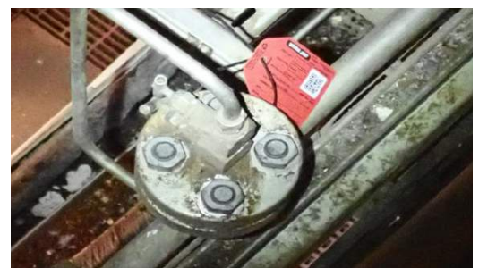
IMAGE SHOWING THE REPLACEMENT OF BOLTS FOLLOWING THE UTILISATION OF THE KLINGER FLANGE TOOL
