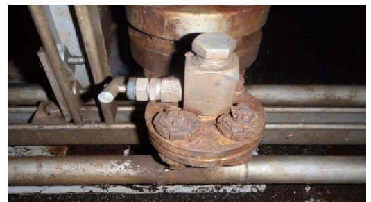
IMAGE SHOWING TYPICAL CORROSION ON BOLTS BEFORE REMOVAL ON 150# FLANGES
